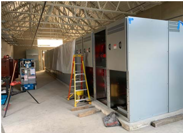
Substation with switchgear installed
